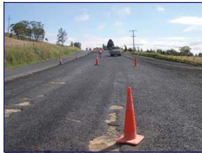
Bonding and Embedment Problems in New Seal
